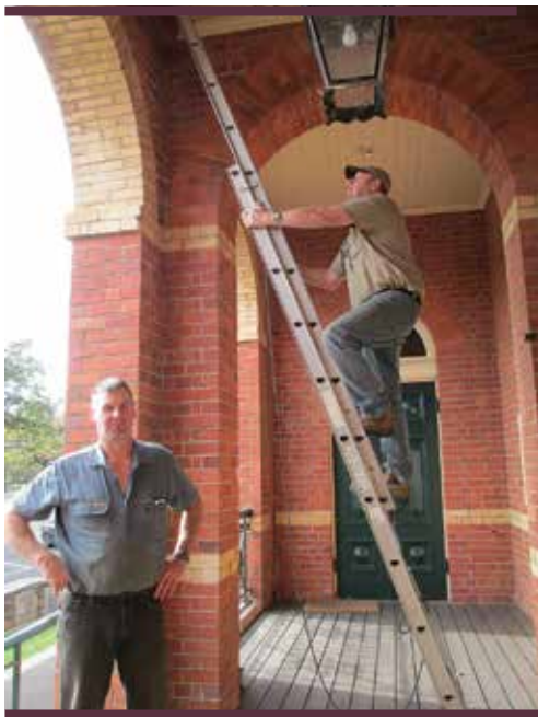
The first stage is for Frank and Chris to access the manhole above the veranda.
