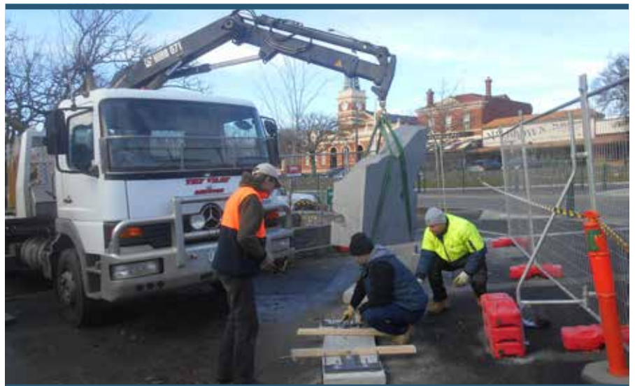
Sculptor Cliff Burttt (left) watches as a section of the sculpture is unloaded and lowered to the base.
