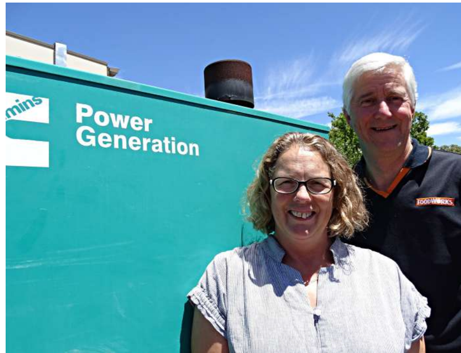
Foodworks' owners Alison and Trevor Rickards' big investment in solar and back-up power is now paying dividends keeping the store open and eliminating stock loss when power fails in the area
